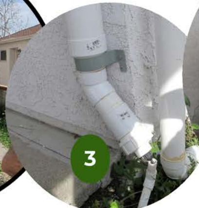
Overflow Drains to Rain Garden
