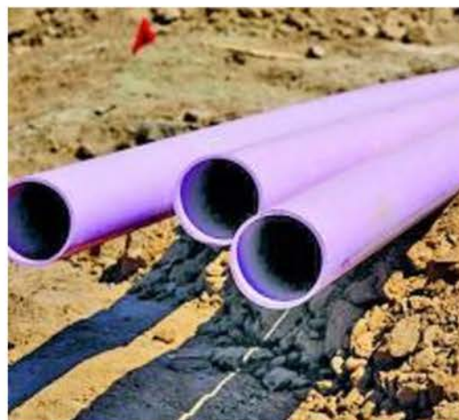
Purple pipe is used to indicate the water is reclaimed.
